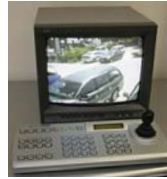
CCTV monitoring system
